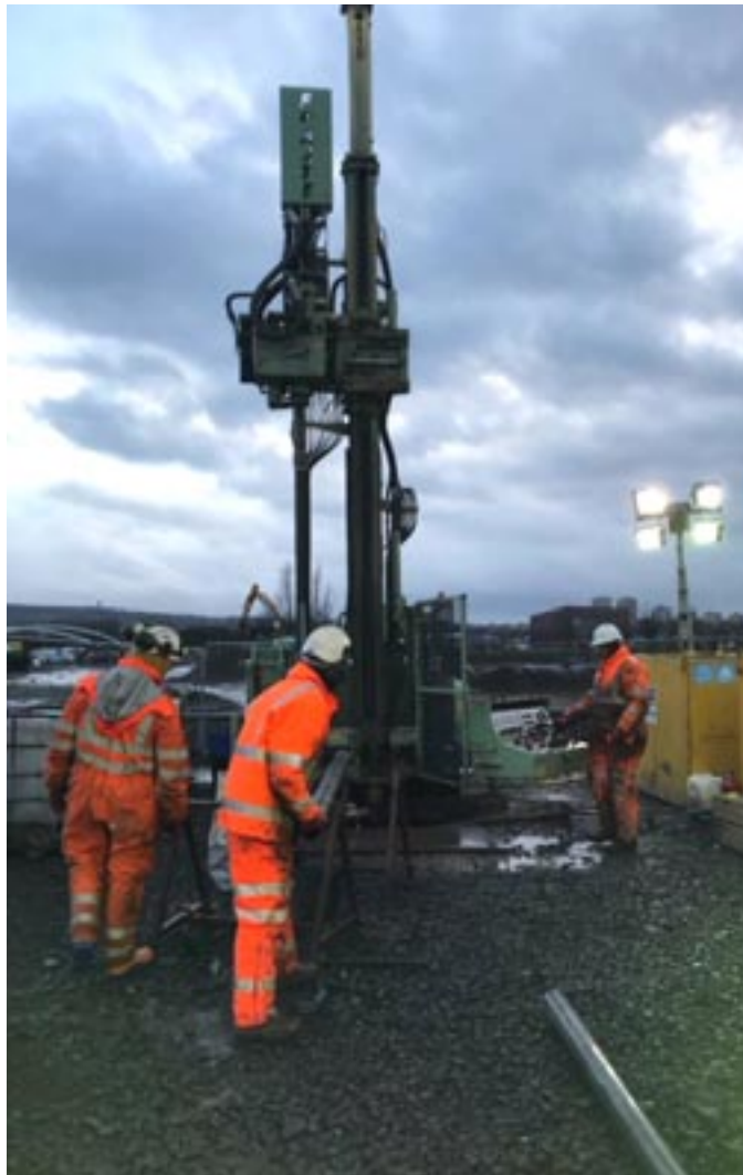
Drilling an observatory in Glasgow to study heat in flooded mineworkings. © Mike Stephenson.
